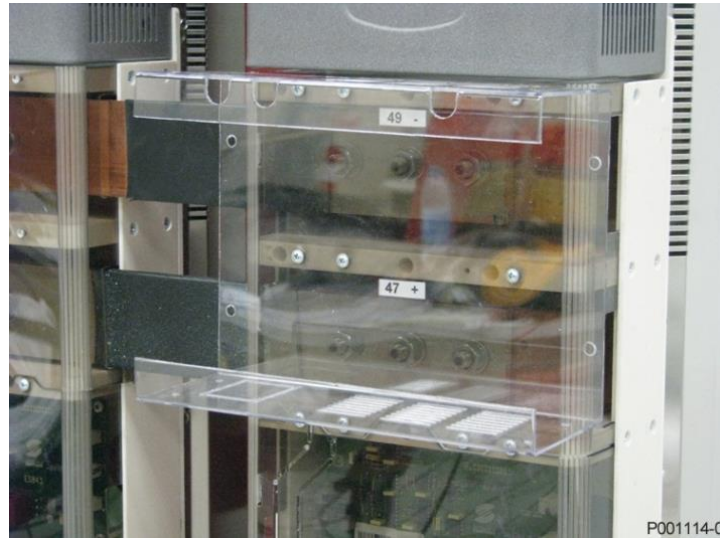
Figure 28: Cable raceway installed on the inverter module
